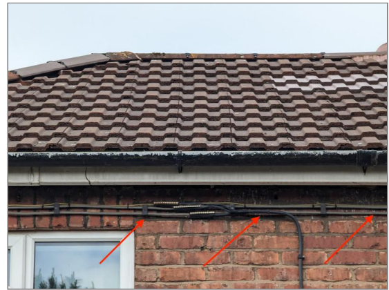
Photo - 40 Electricity cables.
