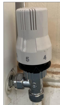
Photo - 46 Thermostatic radiator valve (TRV).
