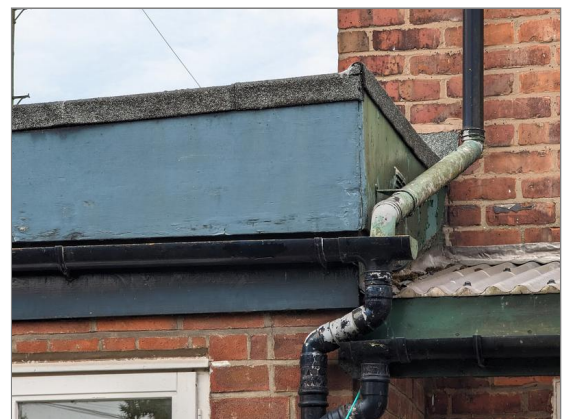
Photo - 24 Timber sections typically weathered
