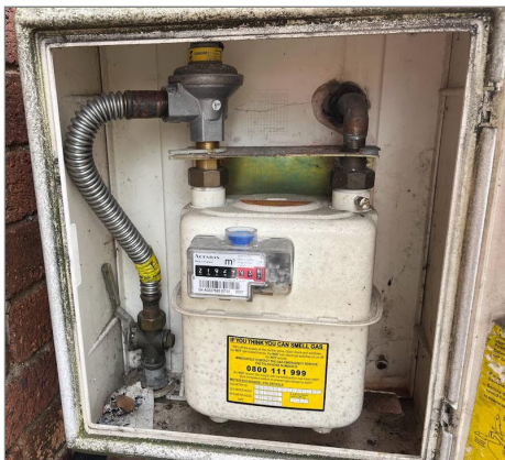
Photo - 41 Gas meter.
