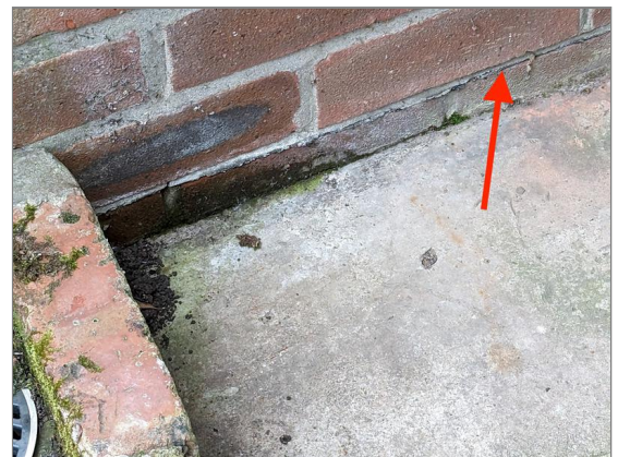
Photo - 14 High ground levels - bridging DPC - create soakaway
