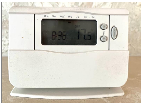
Photo - 45 Boiler programmer and room thermostat.
