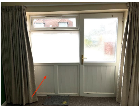
Photo - 38 PVC wall prone to condensation and heat loss.
