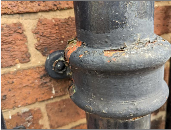
Photo - 49 Typically rusted in places
