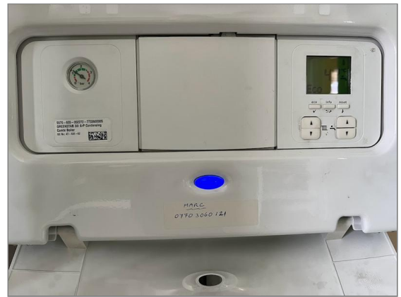
Photo - 44 Boiler control panel.
