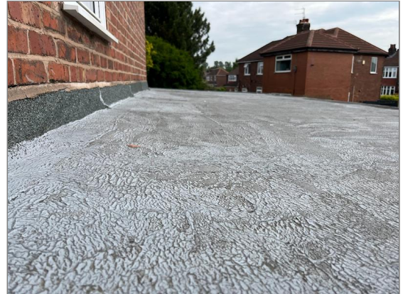
Photo - 6 Flat roof covering - weathered.
