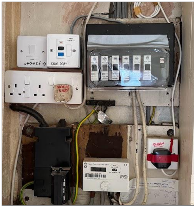
Photo - 39 Dated electrical installation.
