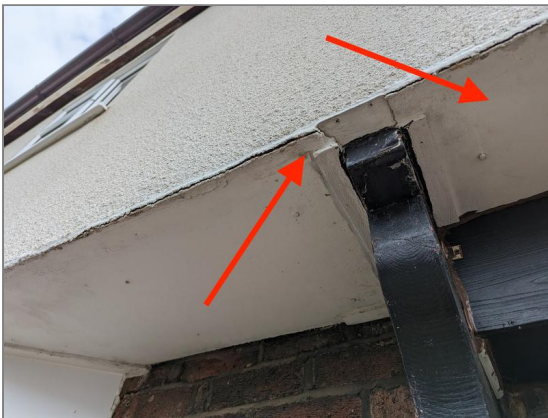
Photo - 17 Possible asbestos content above entrance area
