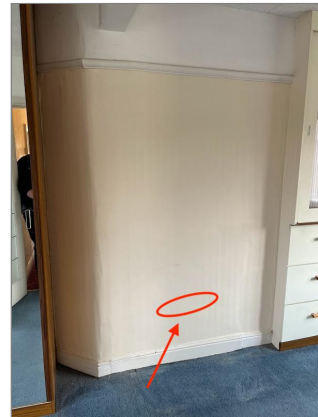
Photo - 34 Chimney breast vent required.
