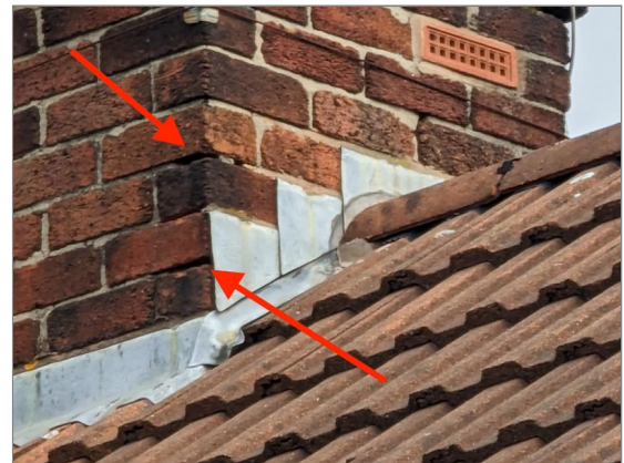
Photo - 2 Localised repointing is now due in some areas
