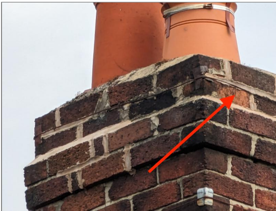
Photo - 3 Weathered brick faces in some places
