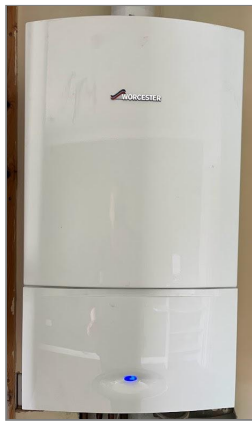
Photo - 43 Central heating boiler.
