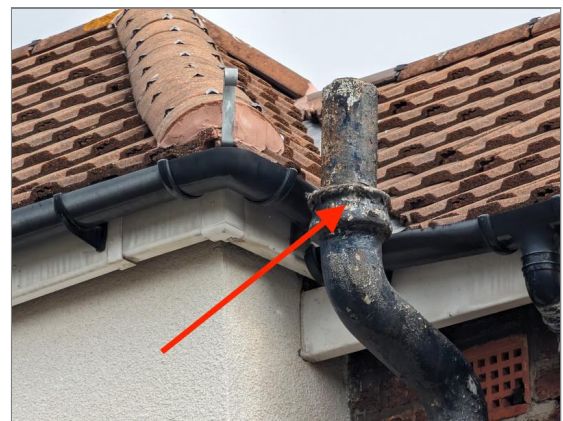
Photo - 48 Dated soil pipe consider replacement
