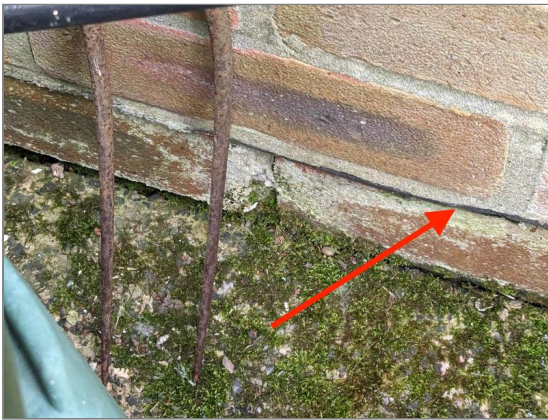
Photo - 15 High ground levels - bridging DPC - create soakaway
