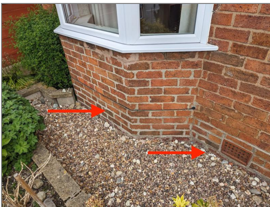
Photo - 13 Create soak-away around all of the external walls (concrete is below the gravel)
