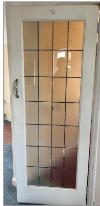
Photo - 35 Glazed internal doors - no safety glass.
