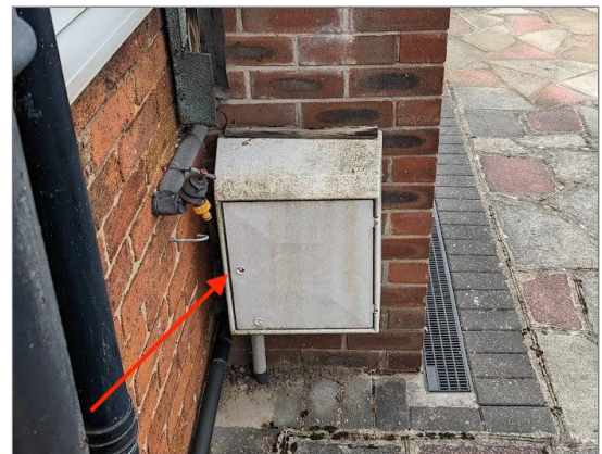
Photo - 42 External meter box.
