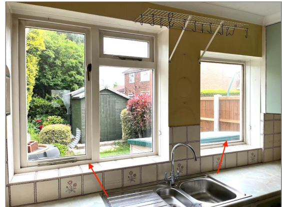
Photo - 19 Dated timber framed windows in kitchen.
