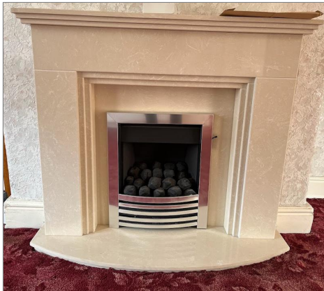
Photo - 33 Living flame gas fire.
