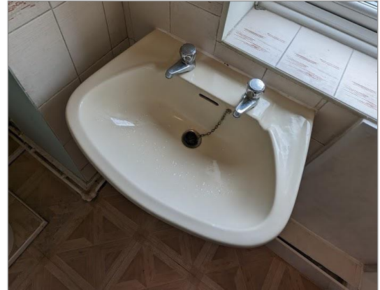
Photo - 37 Basin part of an older installation.
