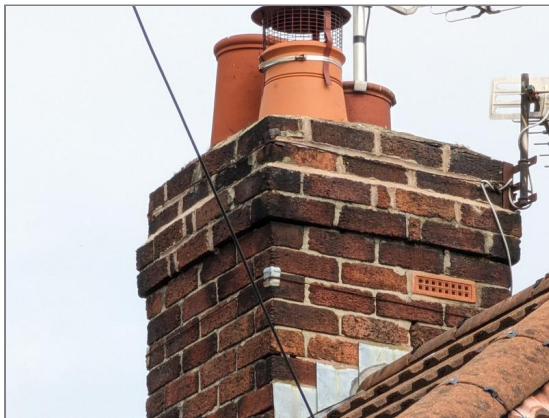
Photo - 1 Front and side face of stack
